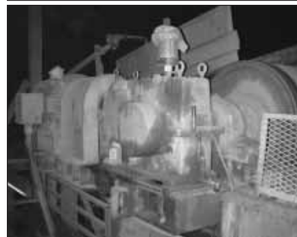
Fig. 8. Gearbox for the 500 ft underground conveyor.
